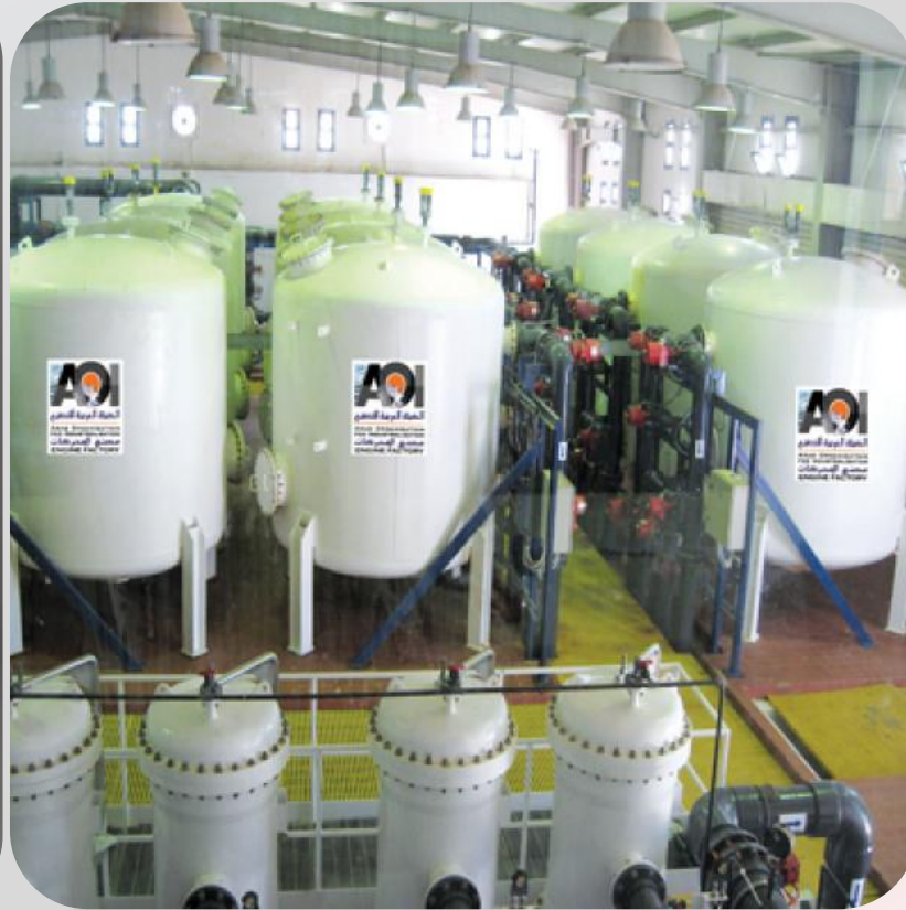
Friendly environment projects such as: Water desalination plants
