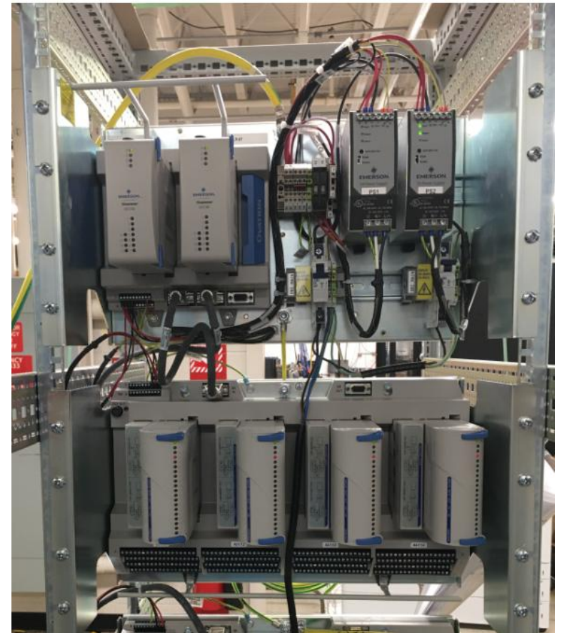
Controllers, Redundant Power Supplies, Horizontal I/O
