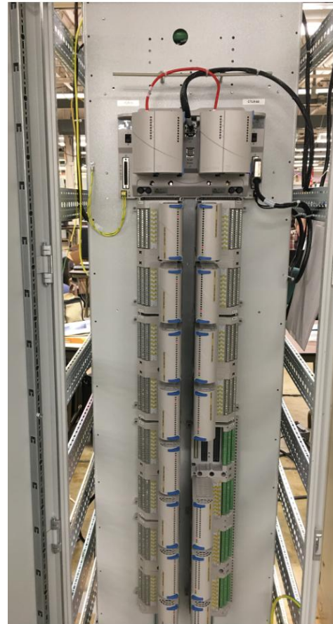
Controllers and Vertical I/O
